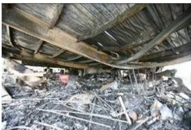
Figure 39 Structural collapse of building
