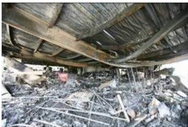
Figure 39 Structural collapse of building
