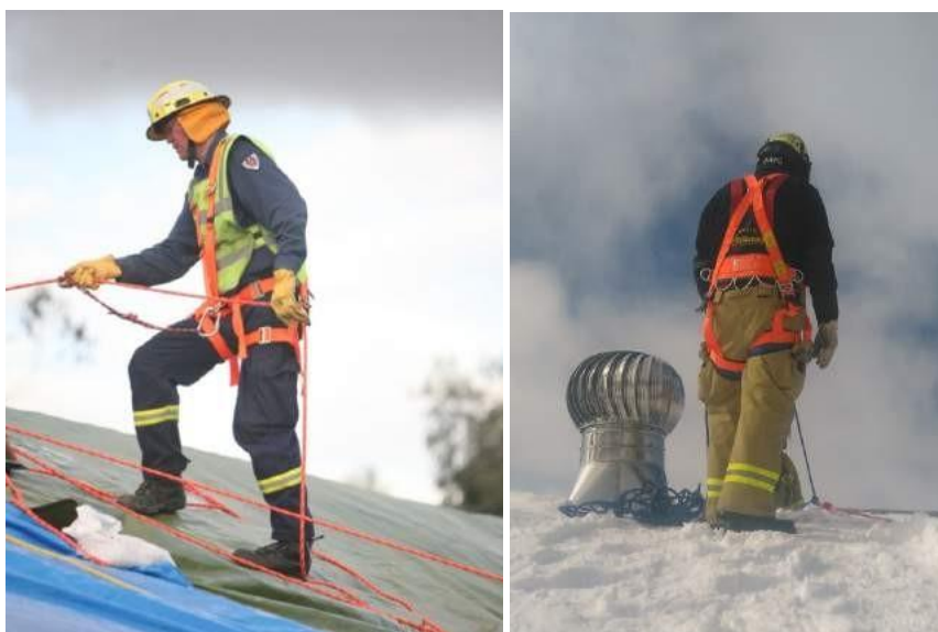
Figure 26 Firefighters working on stormUdamaged roofs
